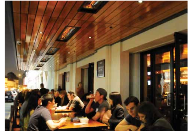
Restaurant with W-Series heaters flush mounted into a wood tongue-and-groove ceiling
