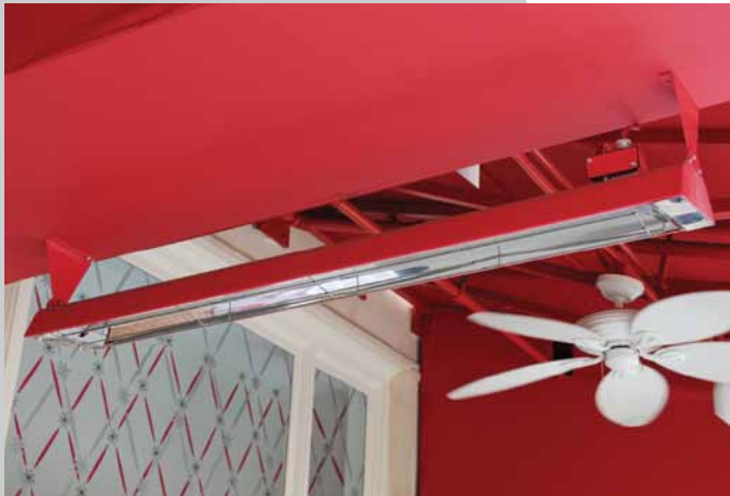
Restaurant patio with custom powder-coated ceiling mounted W-Series heaters
