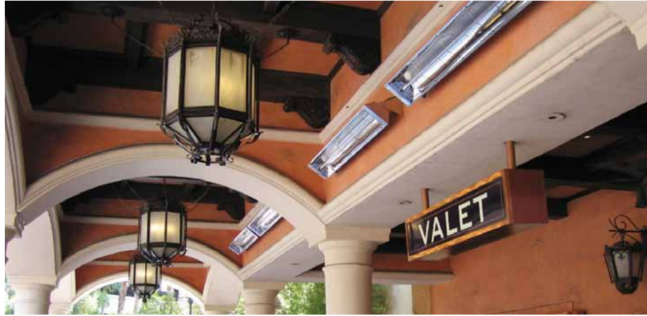
Casino valet station with W-Series heaters wall mounted to a stucco wall
