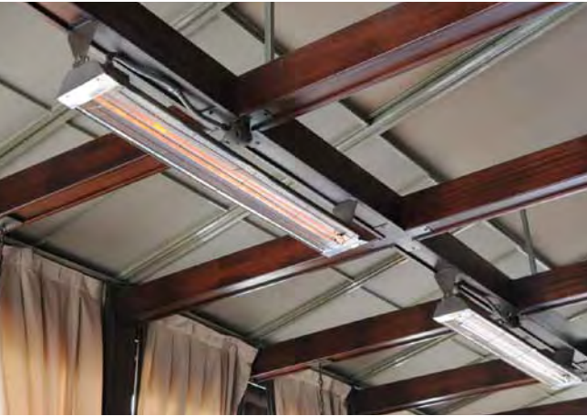
Restaurant with powder-coated bronze W-Series heaters ceiling mounted to a wood beam
